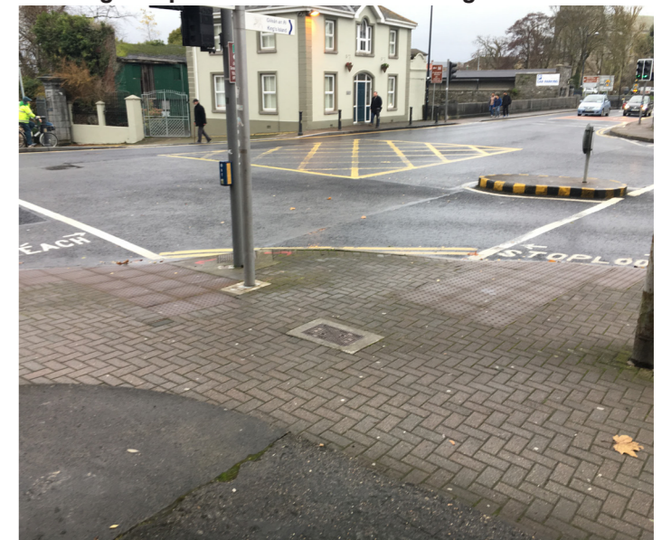
Varied poor paving and non-compliant hazard paving
